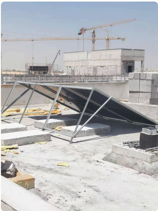
Daytime construction site power supply 白天工地现场供电
